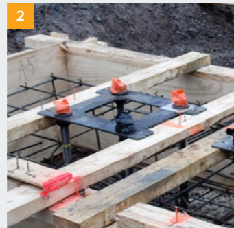
2 Position the PPL template with anchor bolts to the foundation and cast.
