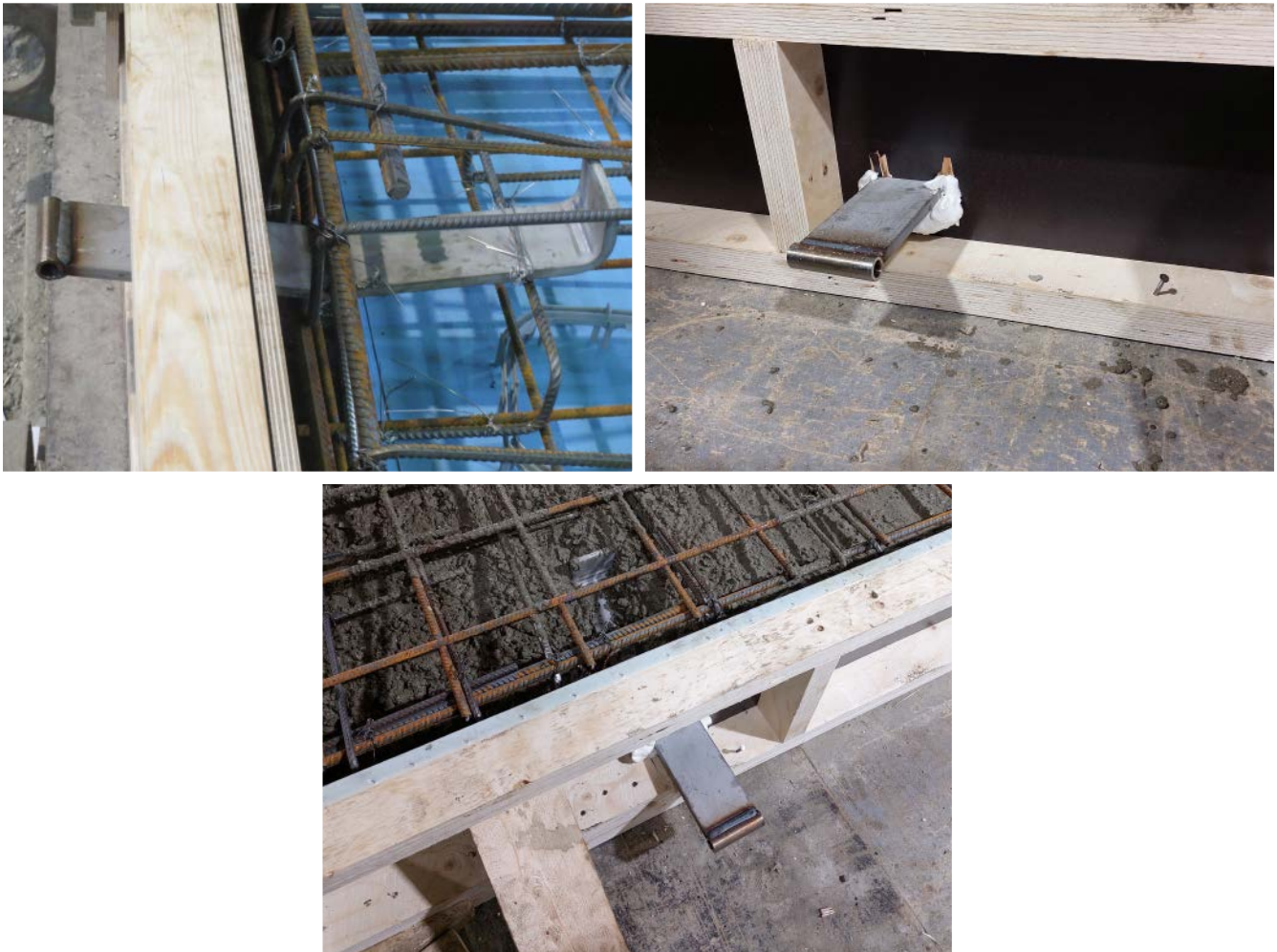
Figure 12. Installation of the PS Balcony Slab Connector Part B to wooden formwork.
