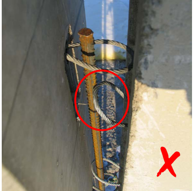
Wrong position of the loop, outside of rebar, short transverse bar
