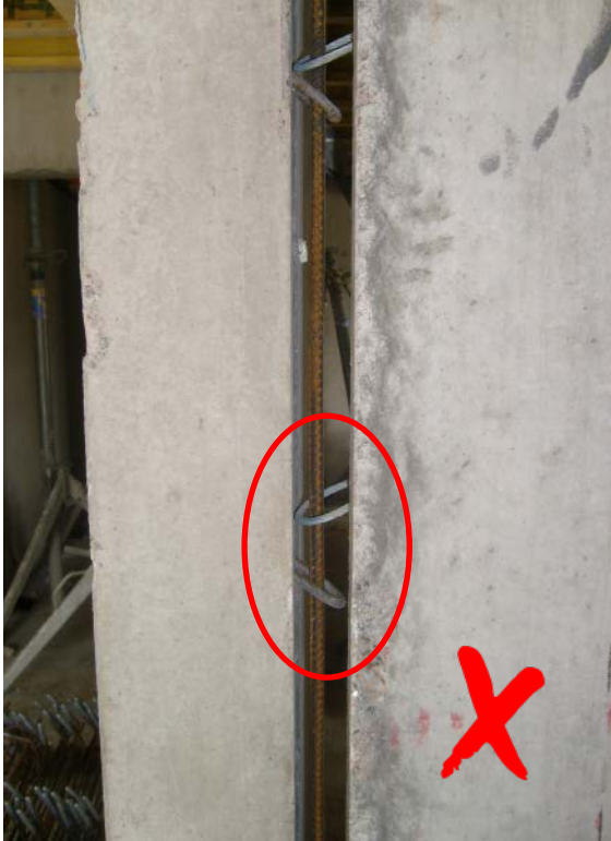
Figure 21. Incorrect installation of wire loops. Spacing between loops is bigger than 20 mm
