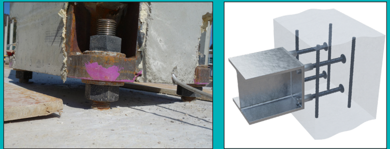
Figure 3. Bolted precast column connection with a gap (left) and a connection between a steel member and THRELDA® Anchor plate (right).
