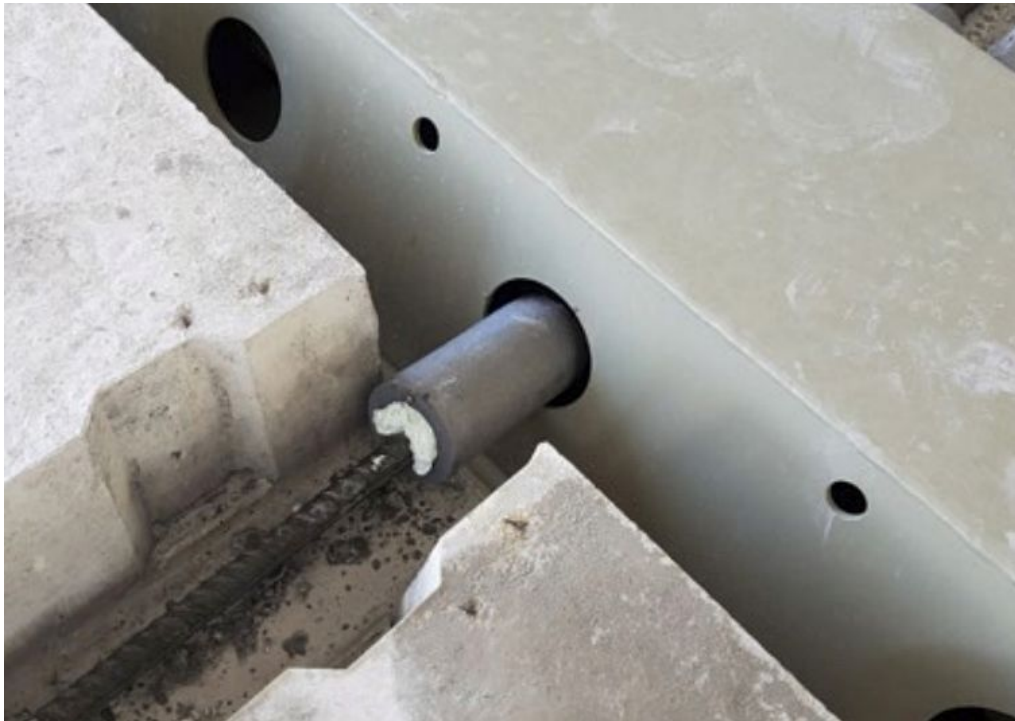
Fig. 5 The rebars connecting the floor slabs through the web holes can be disconnected later on, and then the DELTABEAM® will function as a concrete beam.
