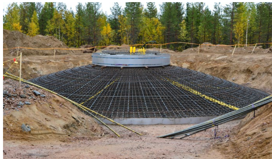
In Lehtirova, Sweden, 41 gravity foundations have been built with a rate of 3 foundations a week during the 2017 season.
