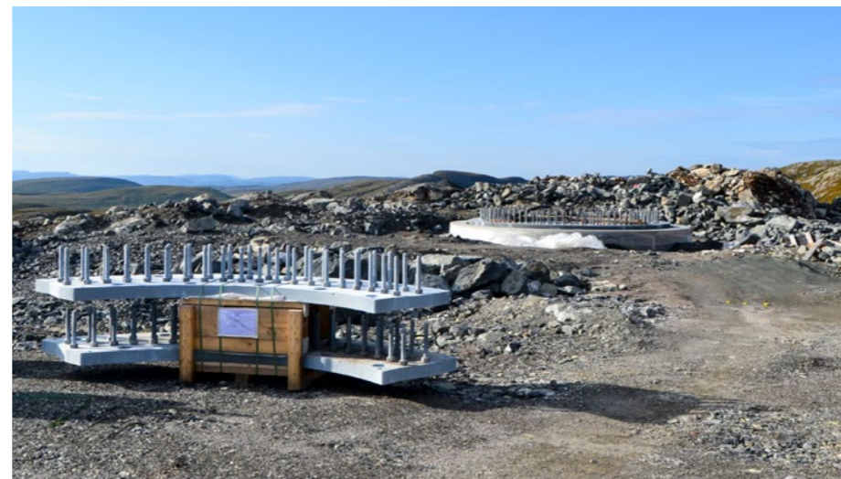
Built in 2017, the Roan site with its 71 rock foundations is a part of the 1,000 MW Fosen Vind project in Norway.
